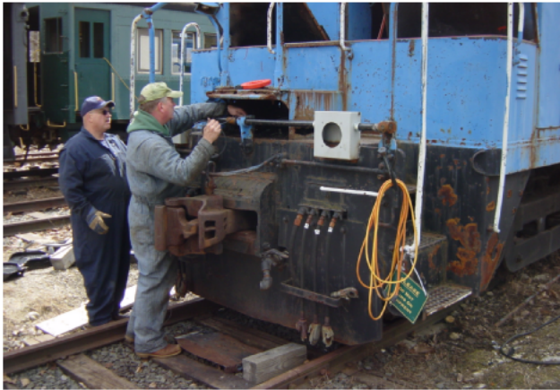
MIKE BOLLOCK AND RICK SELVA PUTTING FINISHING TOUCHES ON DITCH LIGHT WIRING
